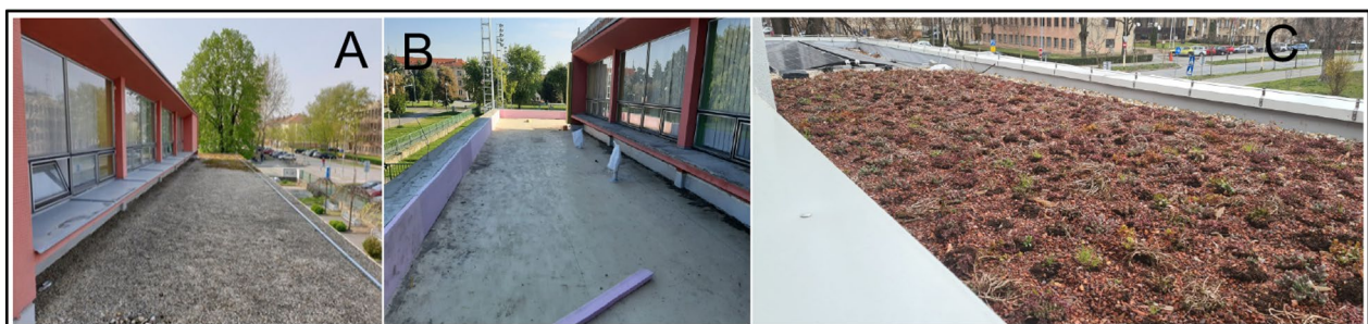
Fig. 4 A Concrete flat roof before energy refurbishment; B construction work in progress during the application of thermal insulation on the flat roof; C green roof after the completion of energy refurbishment
